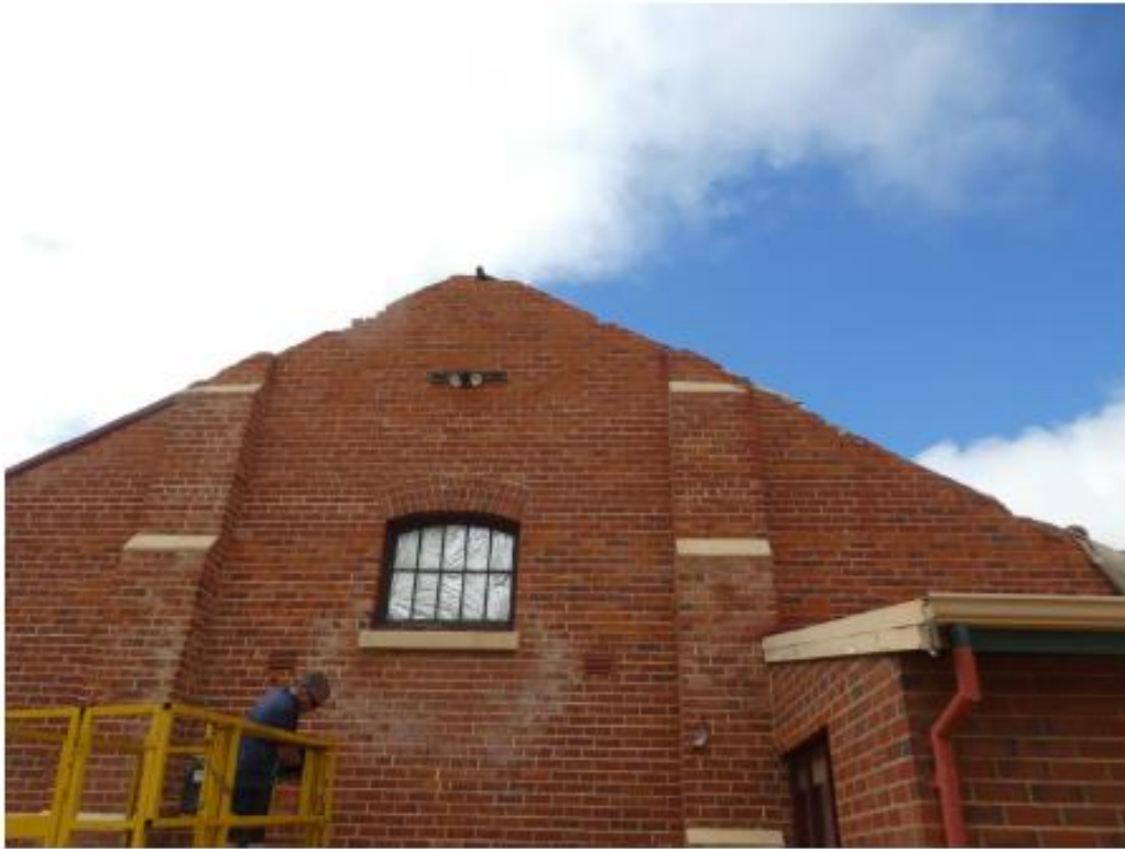
Figure 4: Brickwork at the Top of the Wall needs Repair.
