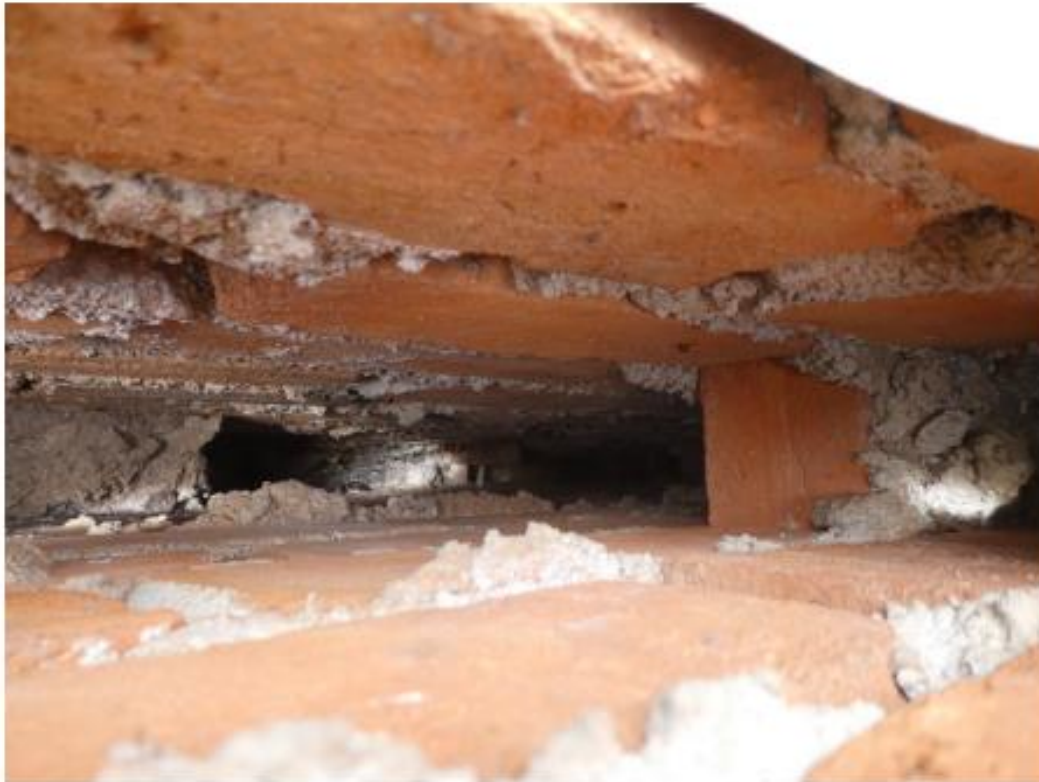
Figure 9; These Cross-Brick Components Probably Saved the End Brick Wall from Blowing Over.
