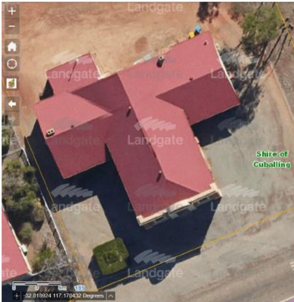
Figure 1; Aerial Photo of Site. The damage to the roof has occurred over the stage at the north end of the main hall. The ceilings over the stage and main hall have been extensively damaged and are in a dangerous condition.
