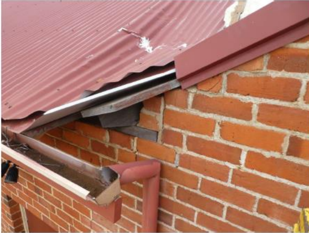
Figure 6; Brickwork at the Top of the Wall Needs Repair.
