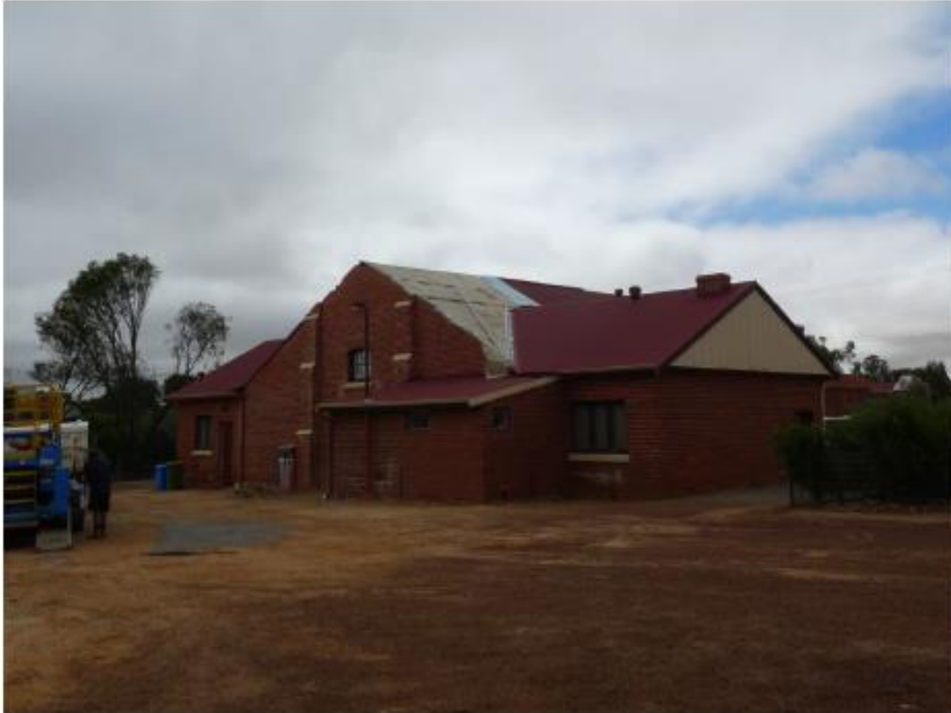
Figure 2; Damage to Northwest side.
