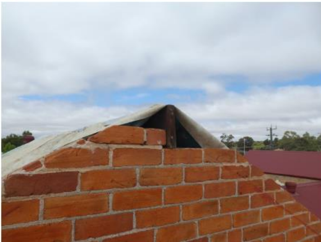
Figure 7: Brickwork at the Top of the Wall Needs Repair.
