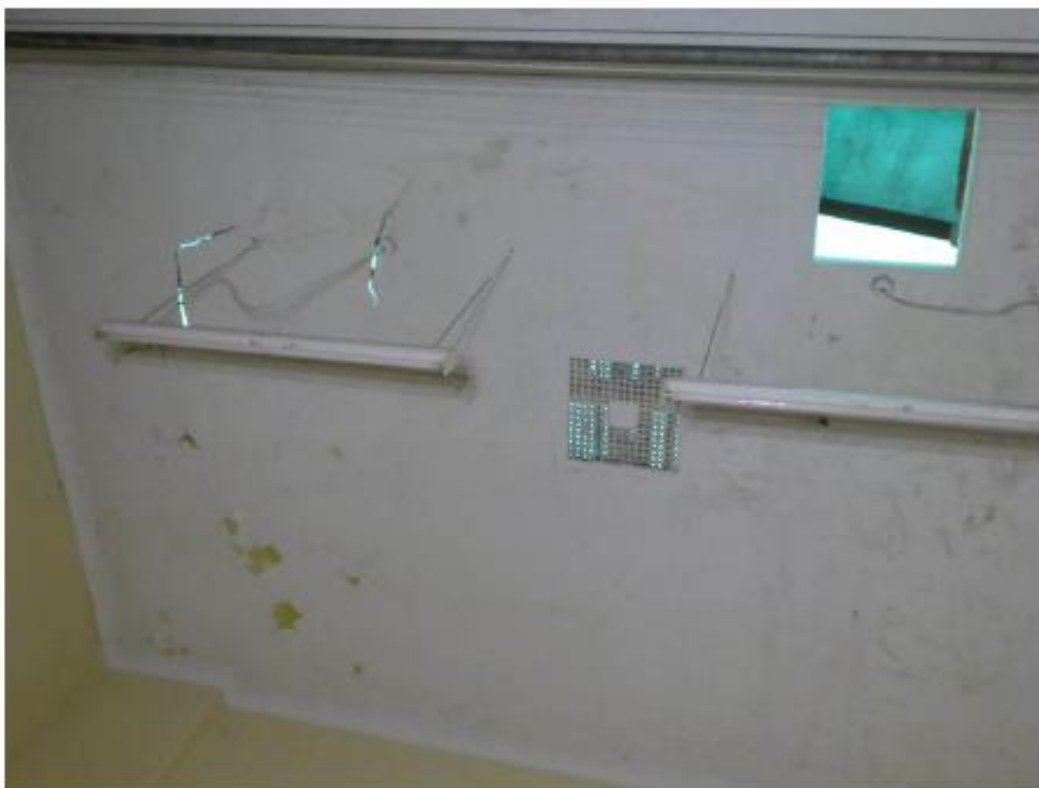
Figure 10; Damage to the Ceiling Over the Stage.
