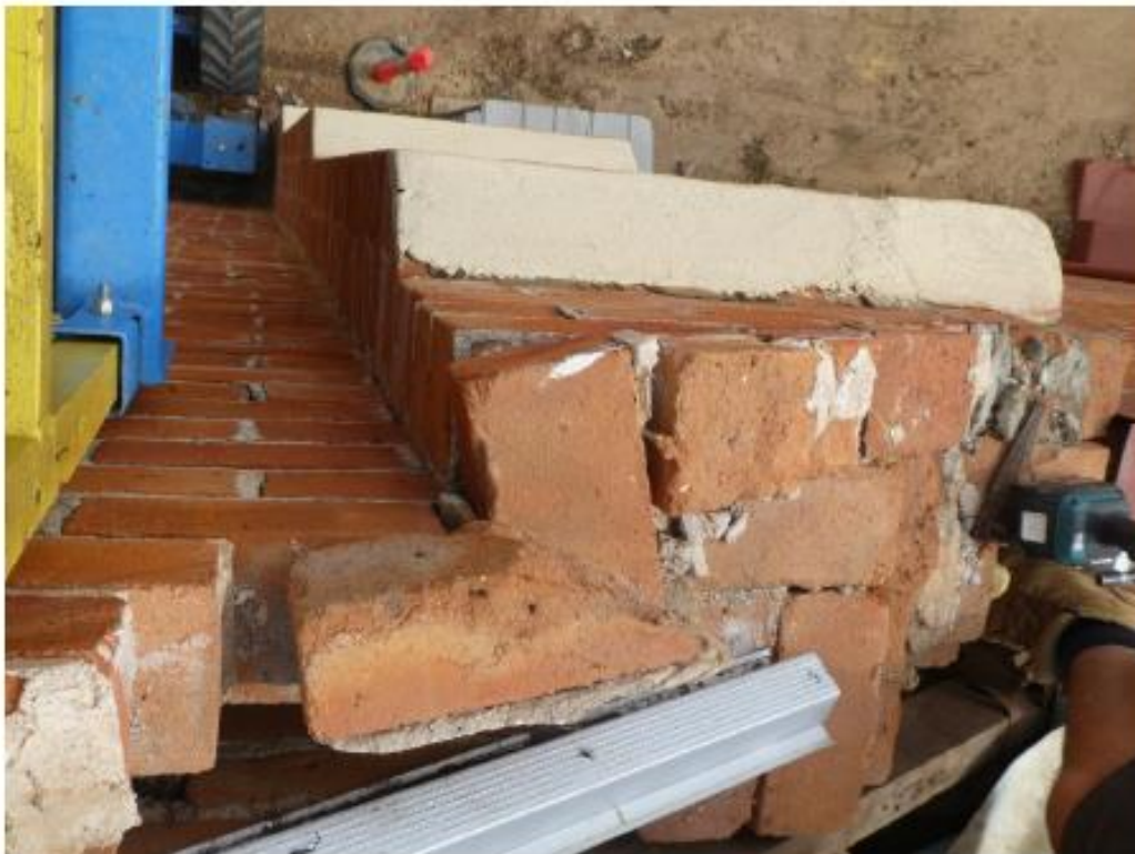
Figure 5: Brickwork at the Top of the Wall Needs Repair.
