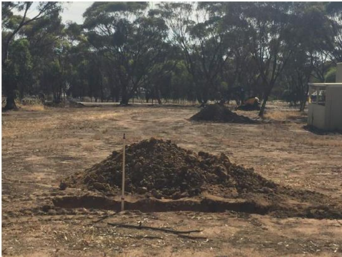
Site Photo showing testholes across Lot 8 – Testhole #1 is in the foreground. Note the BT Mini Excavator in the background.
