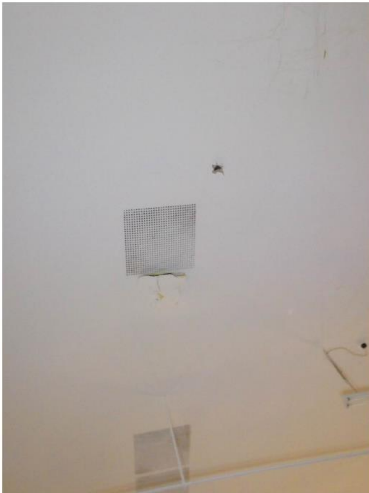
Figure 15; Damage to Ceiling in Main Body of the Hall.
