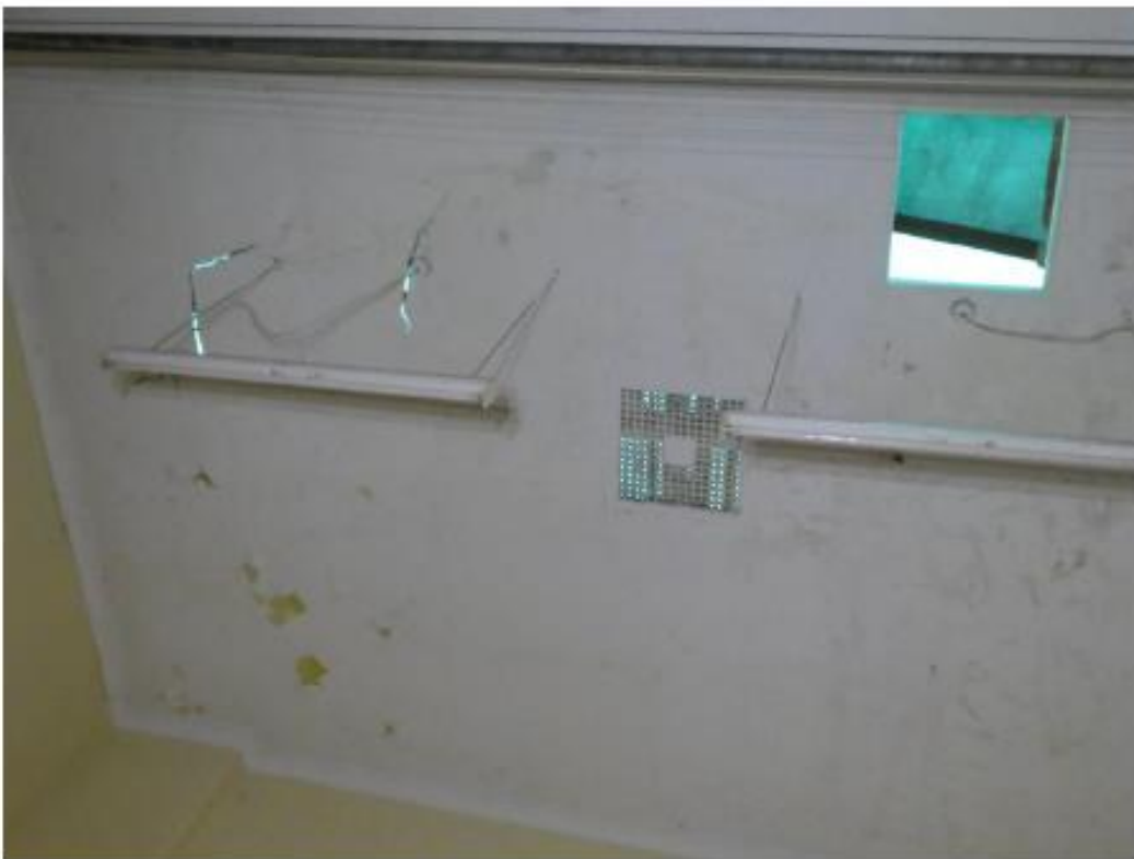
Figure 10; Damage to the Ceiling Over the Stage.
