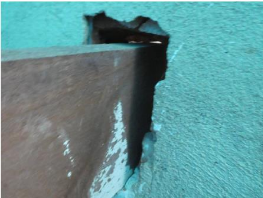
Figure 12: The Hanger Beam Needs to be Fitted into the Wall at the End by Mortaring into Place. It also needs to be fixed at the other end by bolting to timberwork using two 12mm bolts.
