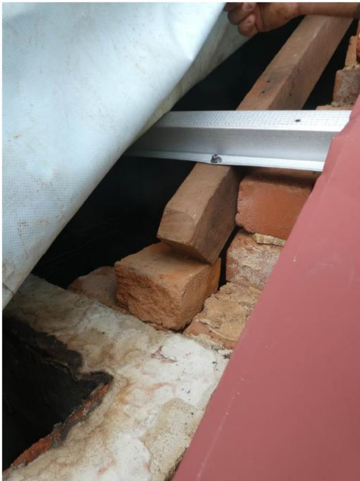
Figure 8; This Rafter needs to be extended and bolted to the Brickwork..
