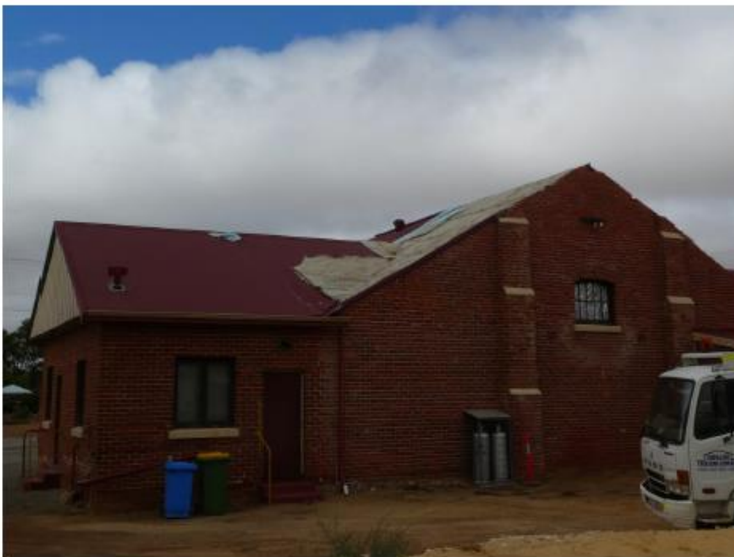
Figure 3; Damage to Northeast side.
