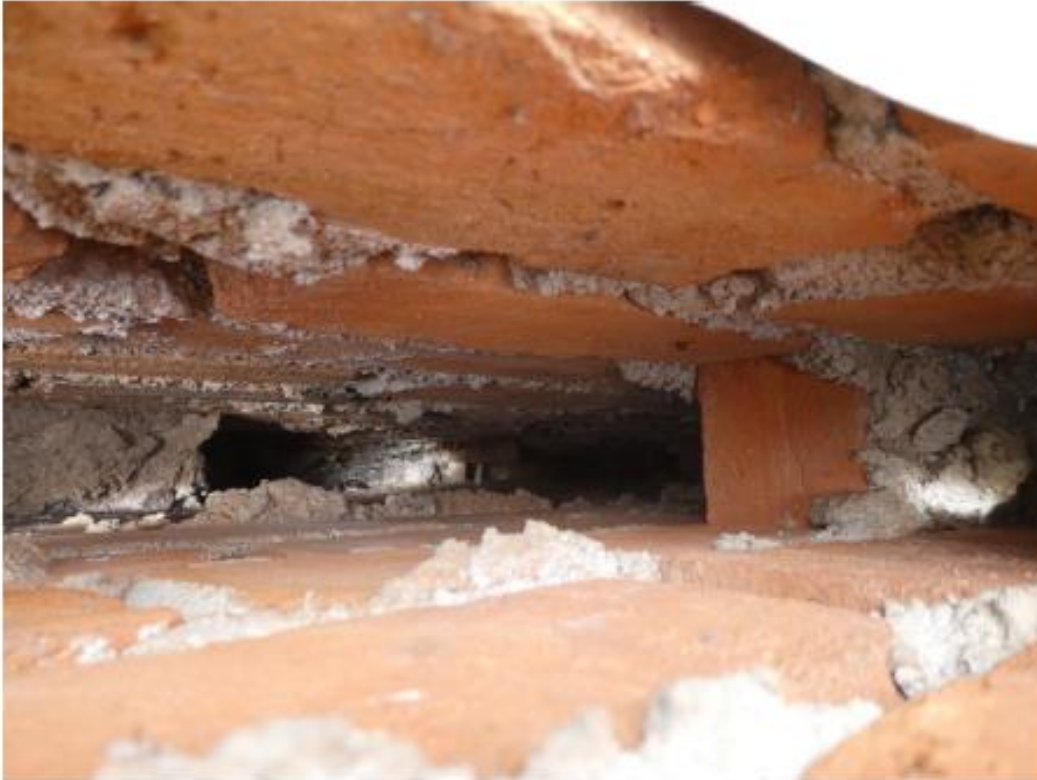
Figure 9; These Cross-Brick Components Probably Saved the End Brick Wall from Blowing Over.
