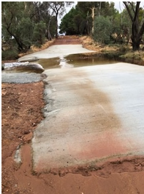
Dent Road Flooding 2022
