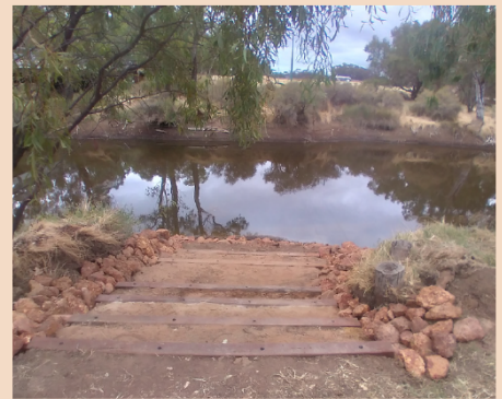
Image: Access steps at Pumphreys Bridge (Works completed by Ben Pike Carpentry)
